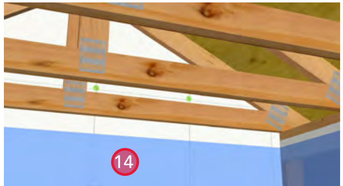
14. Install poly on the walls and fasten to the sheathing membrane with staples.
