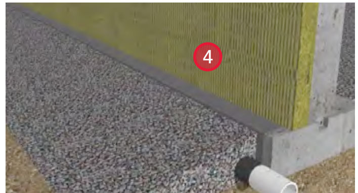
4. Install ROCKWOOL rigid board insulation against foundation wall. Spot adhere the insulation to prevent puncture of the waterproofing membrane.
