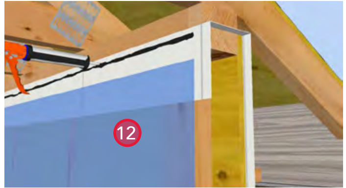
12. Install a bead of acoustical sealant to the sheathing membrane at the lower top plate to transition the air barrier from the wall to the ceiling.
