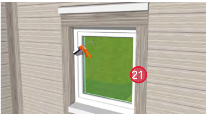
21. Install sealant around the perimeter of the window between the trim boards and the window frame (top and sides).
